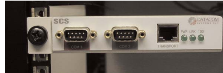
SCS fastened on the left side of the equipment rack
