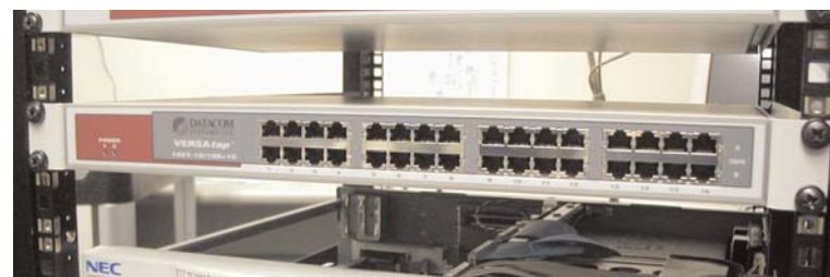
16SY-10/100+1C fastened in the equipment rack
